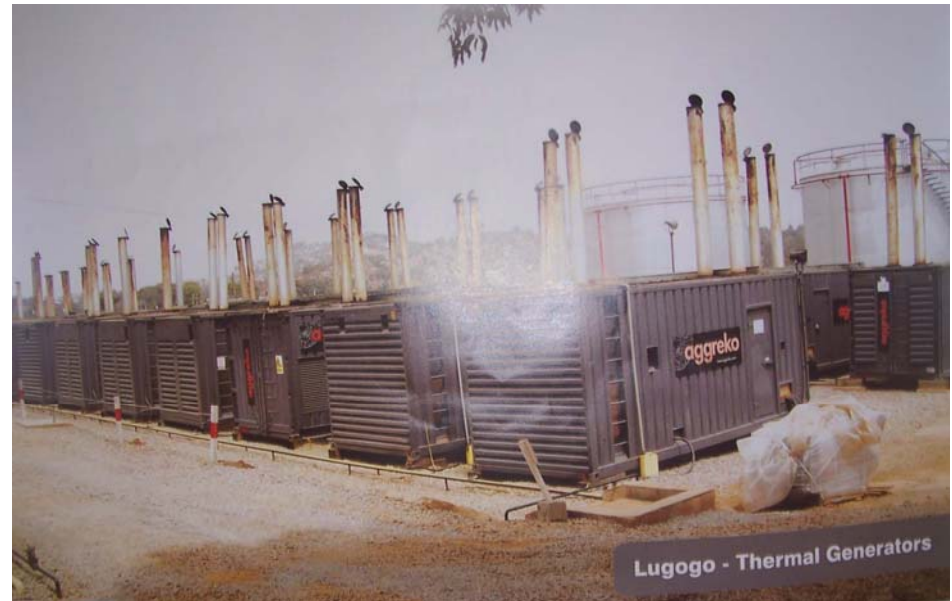
50 MW thermal plant at Lugogo, Kampala
